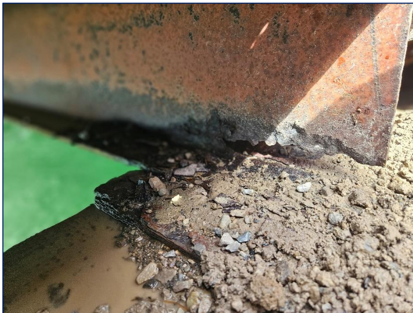
Photograph 8: Severe corrosion and perforation through the lower web at the bearing location on the east abutment. Multiple locations along the east abutment were noted, upon removal of the semi intact ballast wall.
