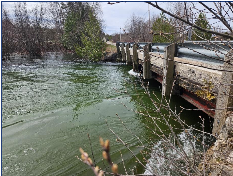
Photograph 20: West elevation with water approximately 16” (400mm) below the underside of the steel beams.
