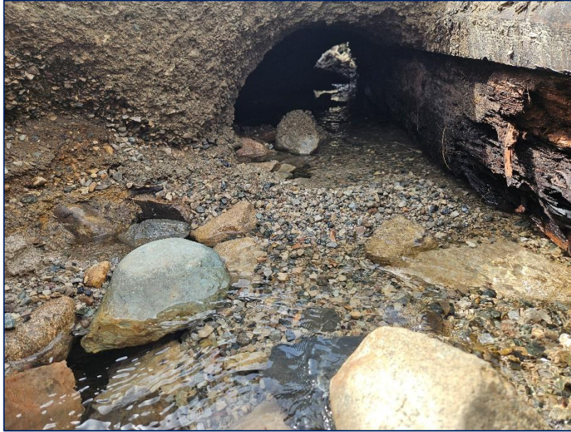
Photograph 7: Looking south along the east abutment/ballast wall at void within the granular backfill. Voids below the wood lagging exist
