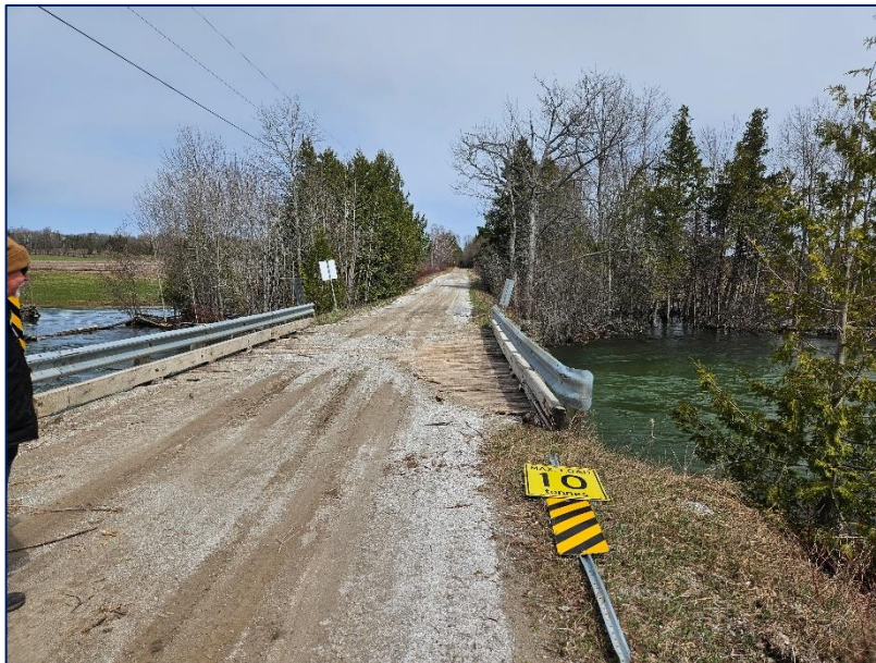
Photograph 16: Looking north across the structure. Gravel on the deck surface has been washed downstream (westerly) indicating extremely high-water levels that overtopped the bridge deck surface.
