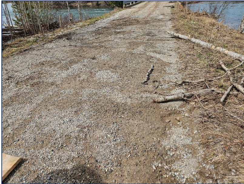
Photograph 15: Looking north towards the structure with wood debris along the roadway and gravel disturbances across the roadway indicating the road was once under water.
