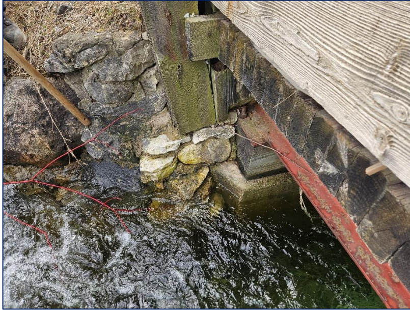
Photograph 23: View of the south abutment bearing timber and contact at the stone/rock wingwall. No signs of any movement of the bridge relative to the abutments.
