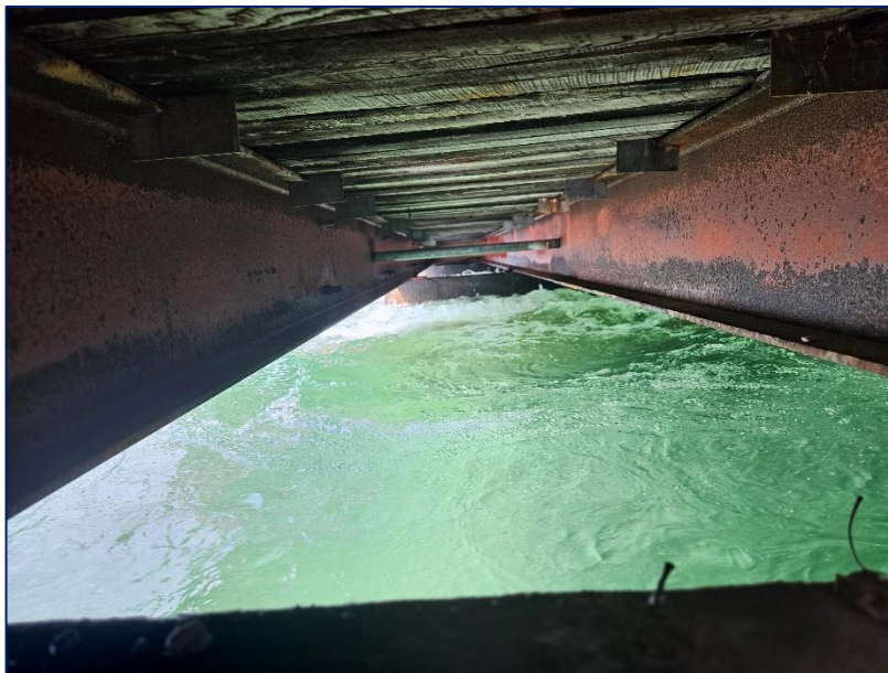
Photograph 12: Looking west from the east abutment along the south exterior beam at the central pier. Steel bracing rods and deck clips are intact.
