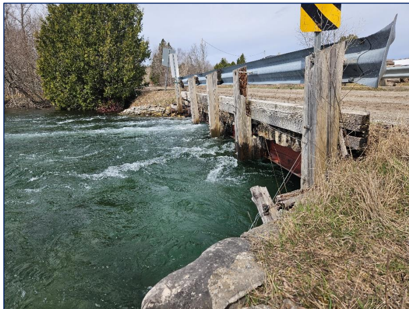
Photograph 4: South elevation – showing high water velocities at downstream end of the bridge.
