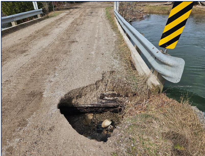
Photograph 6: Typical washout at the east end of the bridge. Voids within the gravel backfill and loss of wooden ballast wall at the ends of the steel beams.
