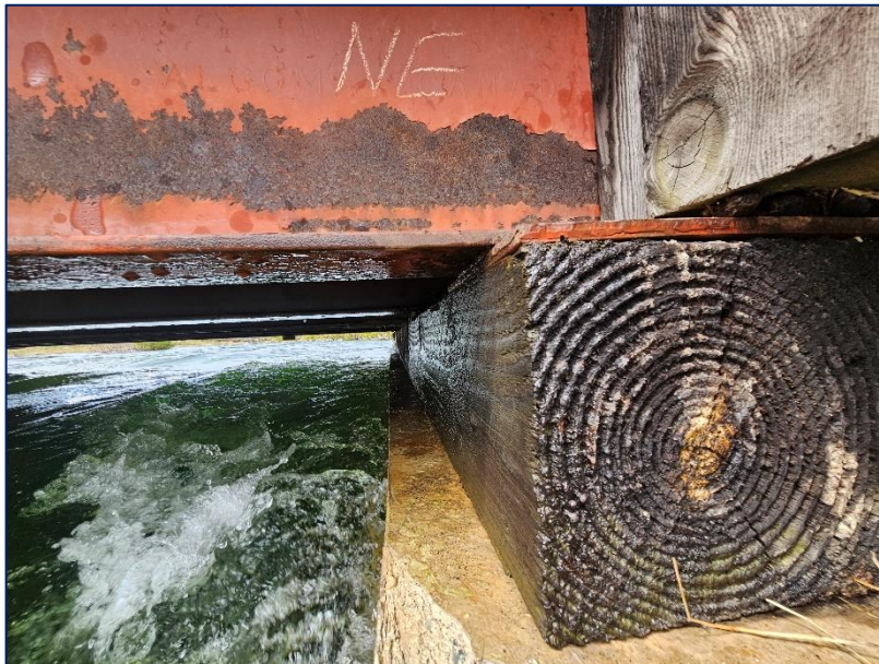
Photograph 24: Looking west along the north abutment at the bearing timber and bearing of the steel beams onto the abutment. Good contact remains with no signs of movements.
