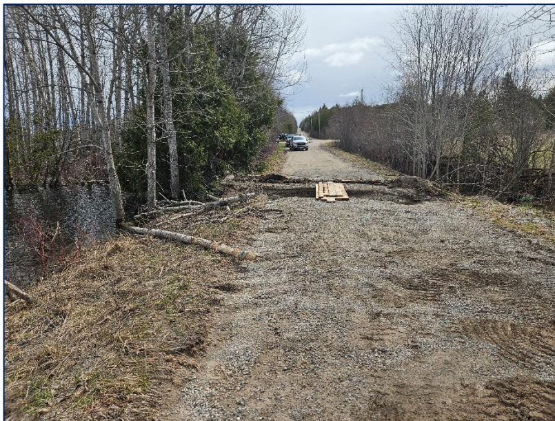
Photograph 2: Looking east along roadway towards the intersection of 2 nd Concession Road and the 20 th Side Road. Wood debris on the roadway, and gravel displacement indicating water had over topped the roadway. Relief channel cut into the roadway by the Township still in place.
