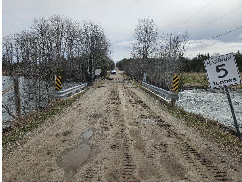
Photograph 5: Looking east across the structure, washouts at the north and south corners of the bridge.
