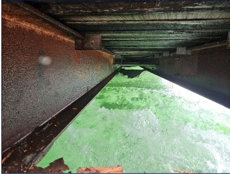
Photograph 11: Looking west at the central pier between the 1 st and 2 nd beams from the north edge of the bridge at the east abutment.
