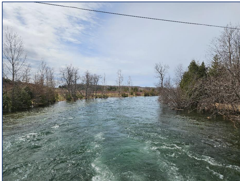
Photograph 14: Looking downstream of bridge site. Water levels have exceeded the normal channel/banks and are pushing into the bush lines along the river.
