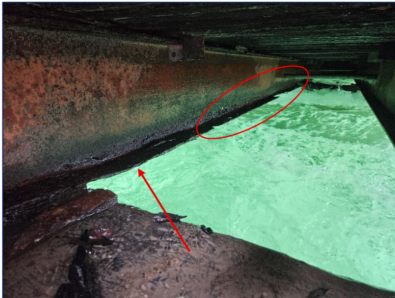
Photograph 10: 3 rd Beam from the North at the East Abutment. Very poor condition with deflection of the bottom beam flange at the abutment and large section loss of flanges out at midspan.
