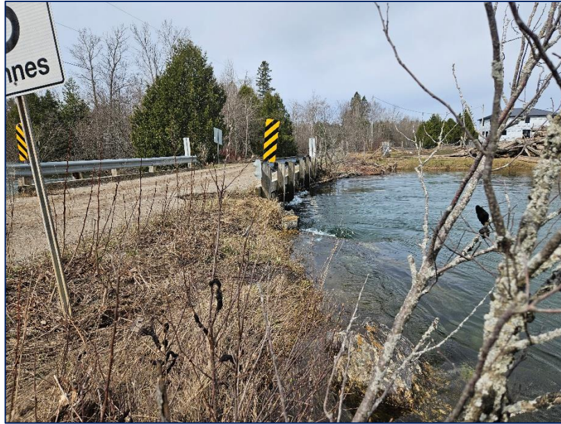
Photograph 3: North elevation – water level was up to the underside of the bridge beams. Washouts in the north and south quadrants of the east abutment.
