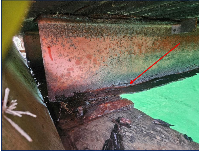
Photograph 9: 3 rd Beam from the North at the East Abutment. Very poor condition, with severe corrosion and major section loss of flanges and lower web.
