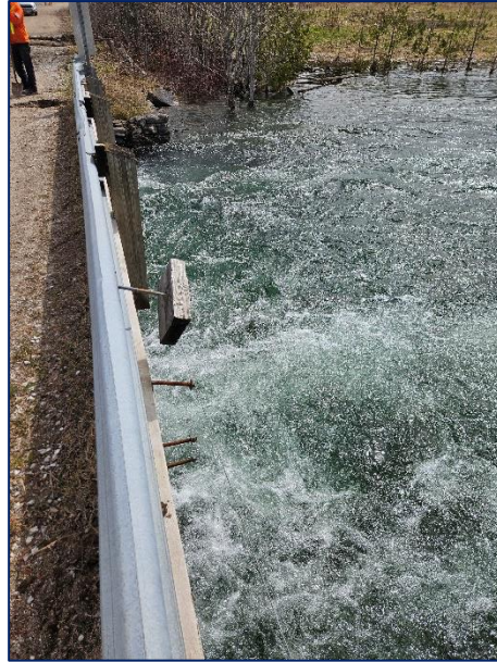
Photograph 13: Missing Guiderail Post on the south Railing system.
